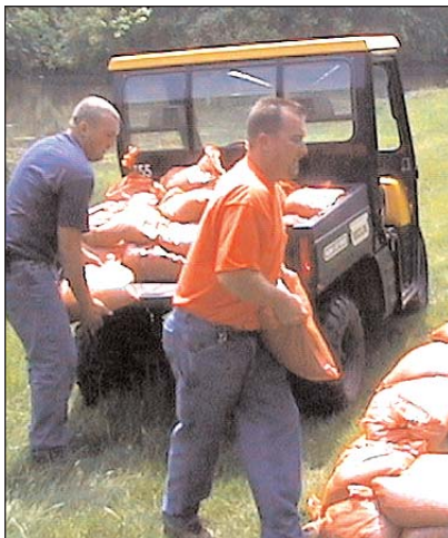
Public Works employees Ed Wegner and Chris Brown (left to right) protect an electrical vault with sandbags in the Shadow Bend Subdivision in anticipation of flood waters that for the most part never materialized.
